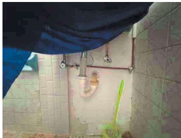
Hot & Cold Water Lines
