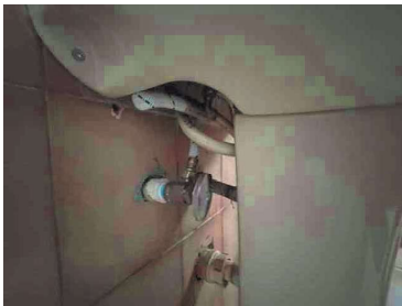
Hot & Cold Water Lines
