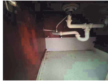
Hot & Cold Water Lines
