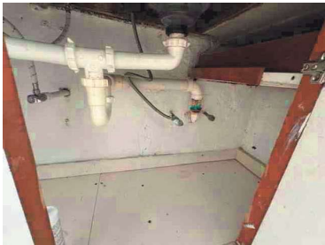
Hot & Cold Water Lines
