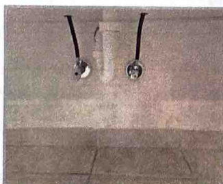
Hot & Cold Water Lines
