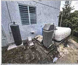
Gas Tank / RWT
