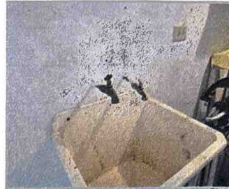
Hot & Cold Water Lines
