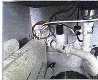
Hot & Cold Water Lines
