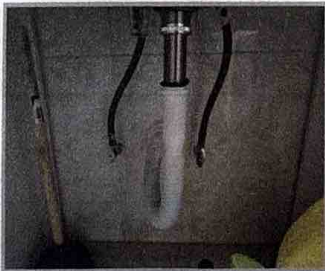
Hot & Cold Water Lines
