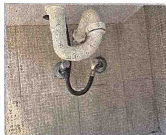
Hot & Cold Water Lines
