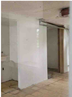
Closet at Ext. Garage
